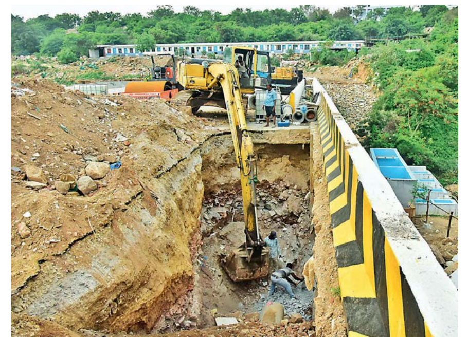
Drainage pipeline works goes on at the new road which was recently completed near ICCB building Road No. 12 in Jubilee Hills. —R. PAVAN
