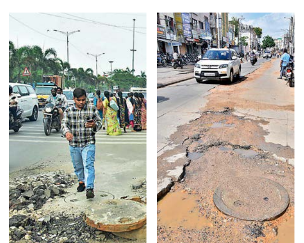
The King Koti to Ramkote Road is dotted with potholes after the Hyderabad Metropolitan Water Supply and Sewerage Board dug up the road for laying pipelines. —P. SURENDRA
