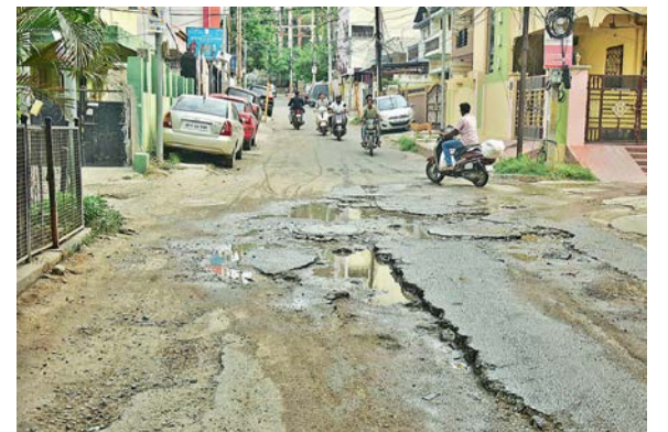
Potholes dot the road at Tolichowki. —DC
