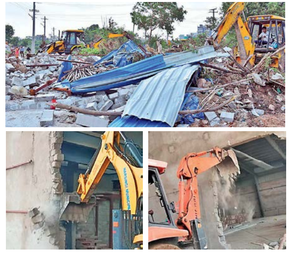
A bulldozer razes a temporary structure at Begumpet. (below) A multi-storey building is demolished in Vattinagulapally. — P. SURENDRA, BY ARRANGEMENT
