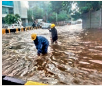
Two workers busy opening the manhole lids for making passage to the rainwater.
