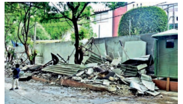
The makeshift structure that was built for security personnel was demolished on Saturday.
