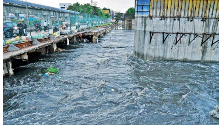
The Musi river is inundated with flood water at Moosarambagh bridge where a new bridge work is in progress. The flood water is almost reaching the level of old bridge on Monday after city witnessed heavy downpour. — P. SURENDRA
