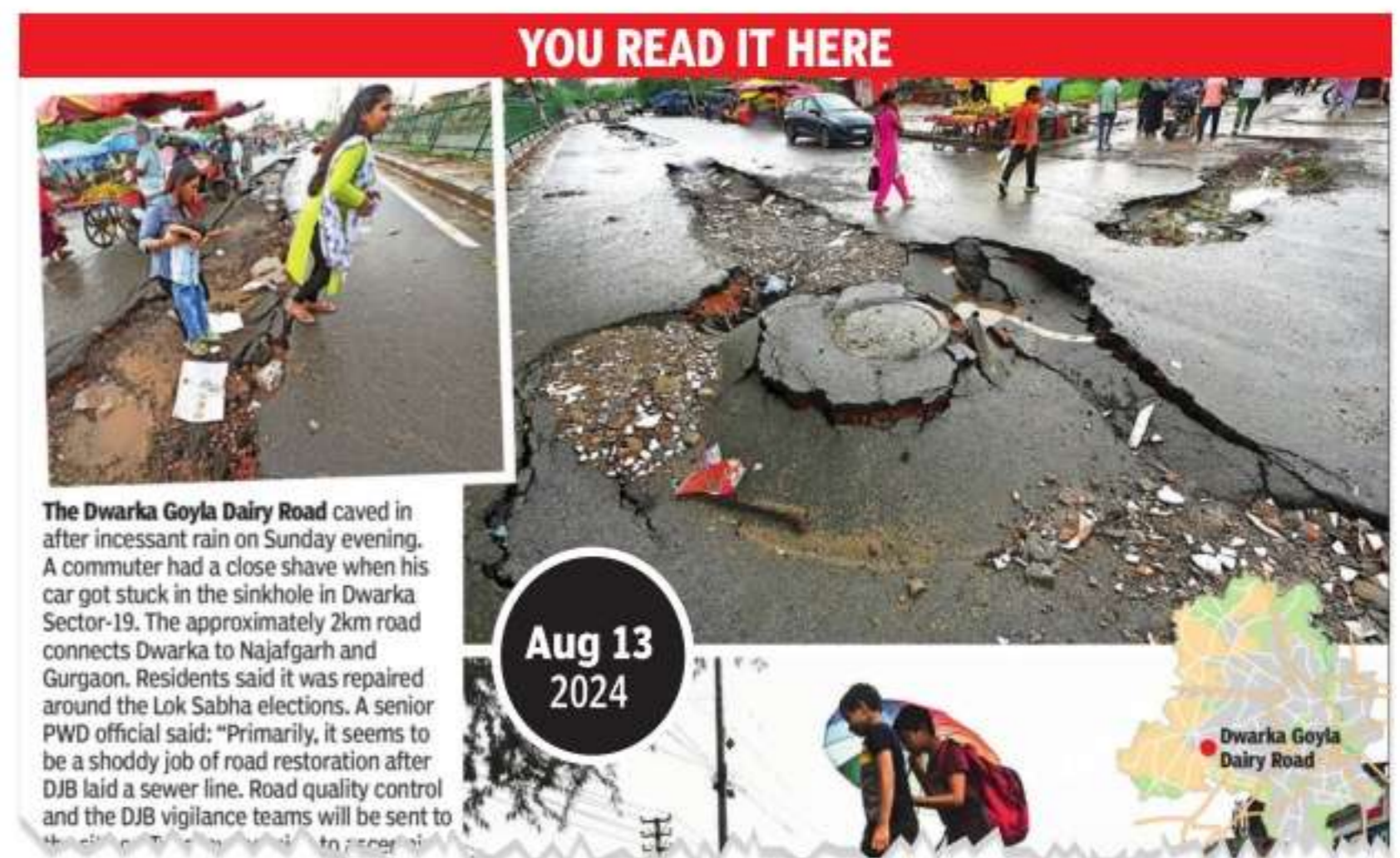
The Dwarka Goyla Dairy Road caved in after incessant rain on Sunday evening. A commuter had a close shave when his car got stuck in the sinkhole in Dwarka Sector-19. The approximately 2km road connects Dwarka to Najafgarh and Gurgaon. Residents said it was repaired around the Lok Sabha elections. A senior PWD official said: "Primarily, it seems to be a shoddy job of road restoration after DJB laid a sewer line. Road quality control and the DJB vigilance teams will be sent to..."
