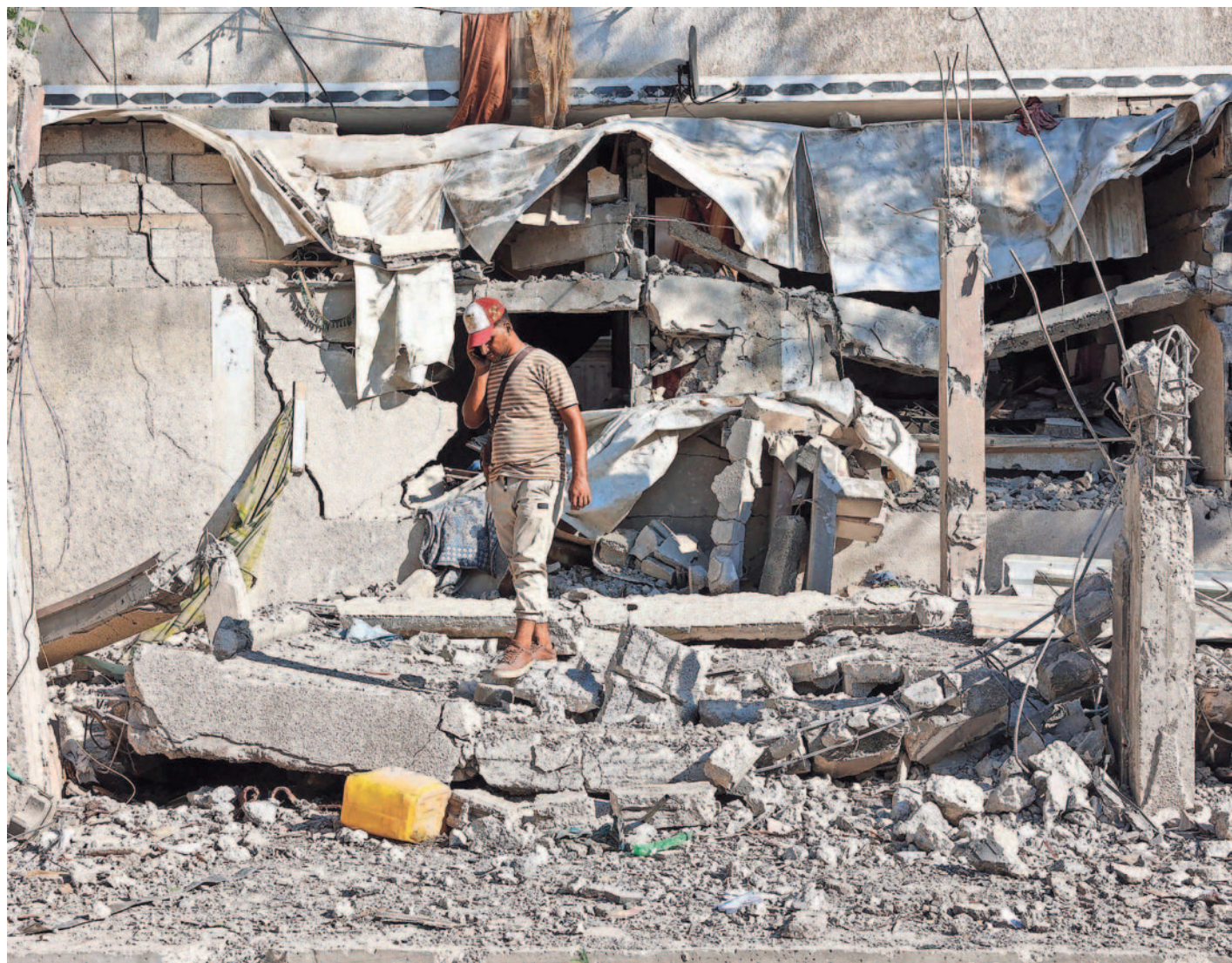
A man inspects the damage following an Israeli strike on Amr Ibn al Aas school housing displaced Palestinians in the Sheikh Radwan neighborhood in Gaza City on Saturday, amid the ongoing war between Israel and the militant Hamas group. The CIA director says detailed cease-fire proposal should be coming this week. OMAR AL-QATTAA/AFP VIA GETTY IMAGES
