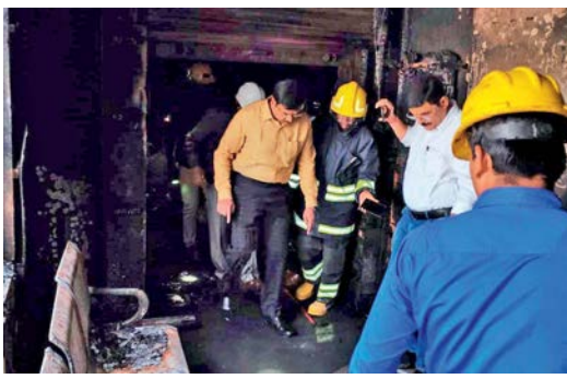
Hydraa chief A.V. Ranganath inspects the Dukes Avenue building in Shaikpet on Friday. — DC
