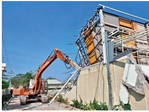
Buildings of Prakruthi Resorts being demolished by HYDRAA on Thursday at Thumkunta Municipality over encroachment of the Komati Kunta lake. — DC
