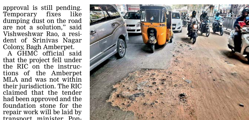
The condition of damaged road at RTC X Roads. — DC
