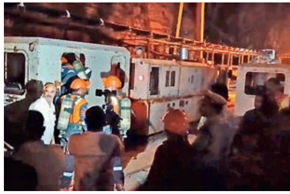
Rescue teams attempt to reach the eight workers trapped in the SLBC tunnel on Saturday. — BY ARRANGEMENT
