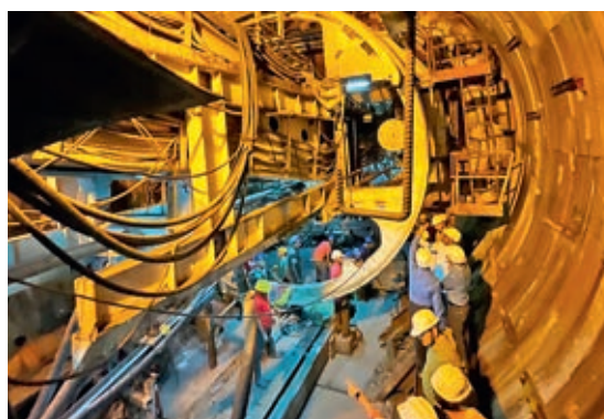
Image shows engineers and operators near the giant tunnel boring machine. — BY SPECIAL ARRANGEMENT
