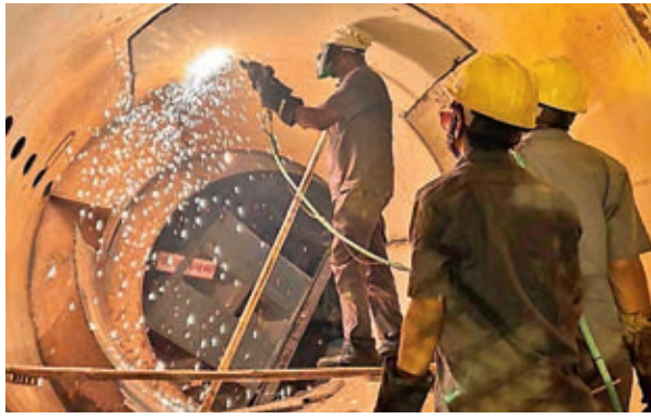
A big hurdle in speeding up the SLBC tunnel clean-up is the broken tunnel boring machine. Efforts to cut it into smaller pieces was on full swing on Saturday. — DC
