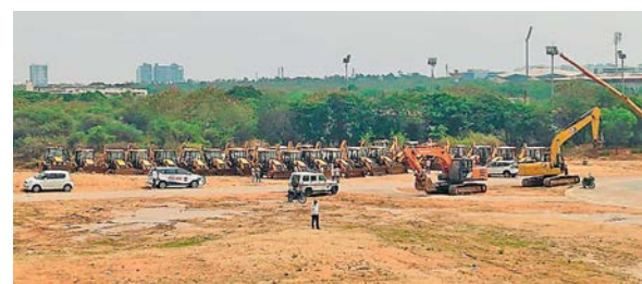
The 400 acres at Gachibowli is being levelled by the authorities, on Monday. — BY ARRANGEMENT
