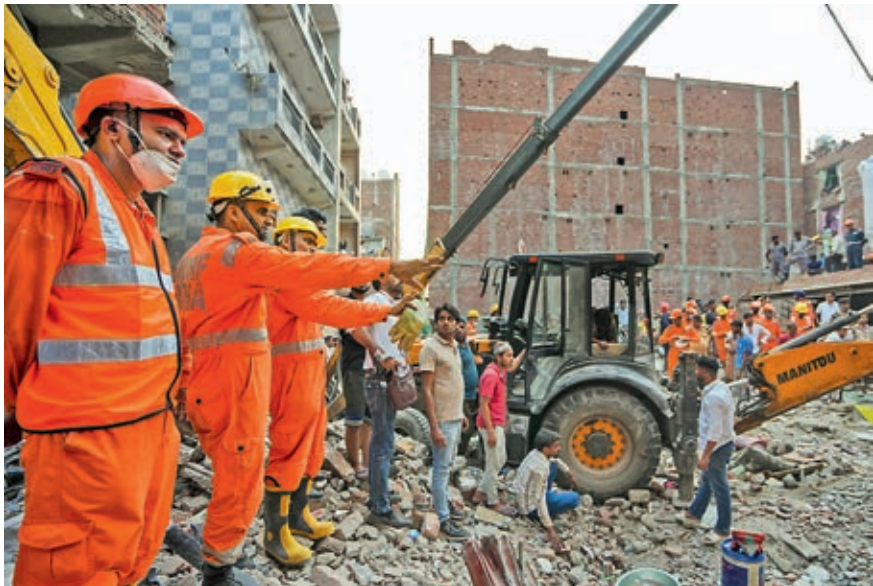
NDRF personnel carry out rescue and relief work after a building collapsed in Mustafabad area in New Delhi, on Saturday. — PTI
