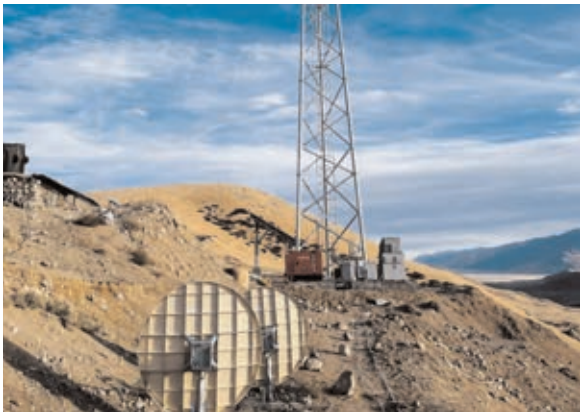
The equipment installed to improve 4G and 5G mobile connectivity to remote regions in high-altitude outposts in Ladakh.
