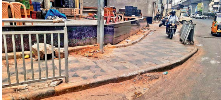
Part of a footpath railing was found removed alleged by traders at Moazzam Jahi Market, Hyderabad, on Thursday, for access to customers but has made it easier for motorists to take a short cut. — P. SURENDRA
