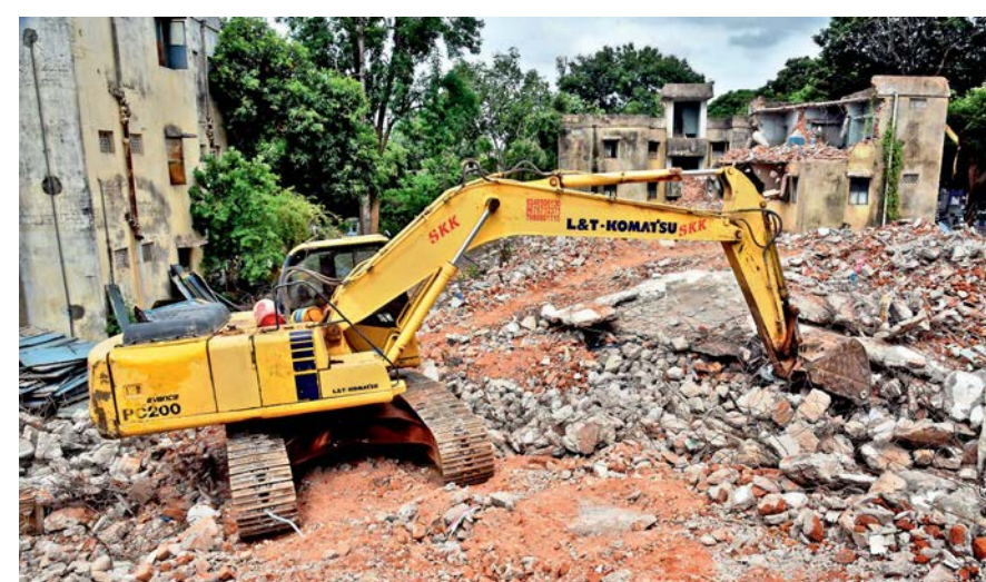
The old police quarters in Begumpet, which was in a dilapidated condition, is being demolished. The quarters was located on the main road. — P. SURENDRA
