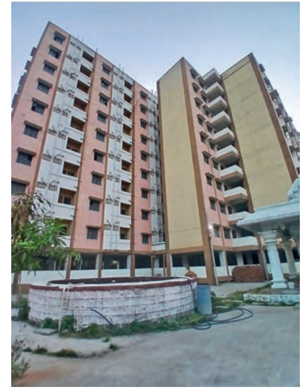
The 2BHK flats at the Dignity Housing Colony in Chilkalguda Dhubighat are yet to be handed over to beneficiaries even after 6 years. The building is getting damaged due to the lack of maintenance. — S. SURENDER REDDY
