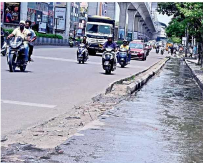
Drainage water overflows onto the service road at Habsiguda, inconveniencing commuters and raising sanitation concerns.
