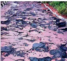
The damaged section of the cycling track on the ORR.
