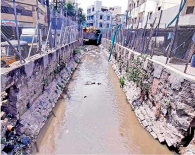
Aghapura nala is now free flow after the Hydra team removed the 56 trucks of loads of garbage which stagnated the flow. — P. SURENDRA
